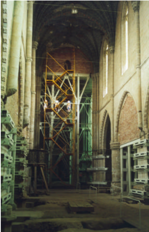
Figure 3: Tarazona Cathedral. Cimborio and clerestory arches propped on steel frame and masonry diaphragms; piers encircled with timber and steel confinement.
